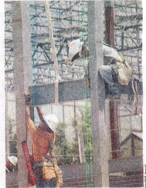
RETAIL ON THE RISE: Steel workers finish out the frame of the new Dave & Busters Restaurant on Walnut Hill and North Central Expressway.
